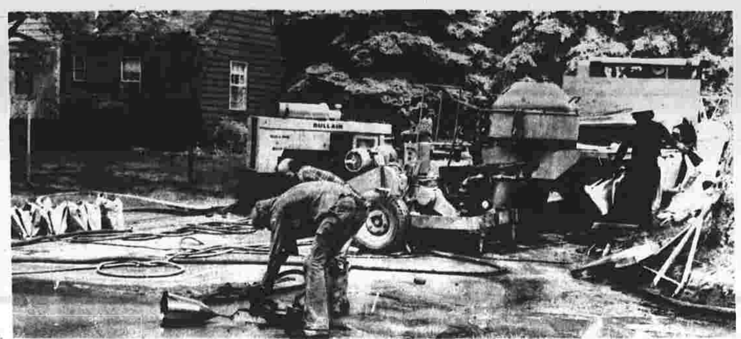
Manchester water work Good weather usually finds construction crews busy throughout Manchester working on a variety of projects.
